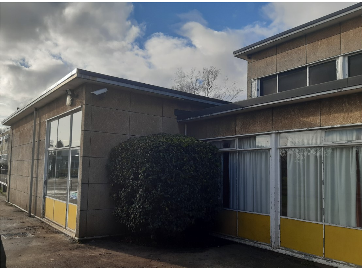
Close up of western range to southern courtyard that shows the original metal glazed screen/fenestration elements and original metal framed windows of the clerestorey to the hall/gym.
